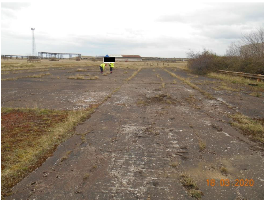
Plate 24 – View looking east southeast showing a hardstanding area. It was noted that the hardstanding surface is ‘wavy’ and cracked, again providing
