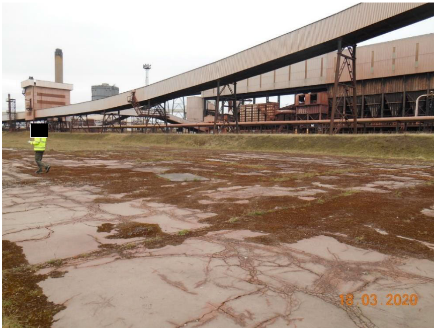
Plate 22 – View looking north west showing area of remnant hardstanding and the Blast Furnace Stockhouse.
