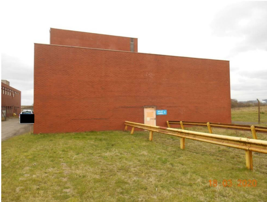
Plate 20 – View looking west showing deformation across the Pellet Tunnel building. It is noted that the extent and direction of the tunnels are not known at the time of this report issue, however STSC have indicated that these records should be available for release. The barriers leading to the structure again delineate the corridor of buried underground services and high voltage cables.
